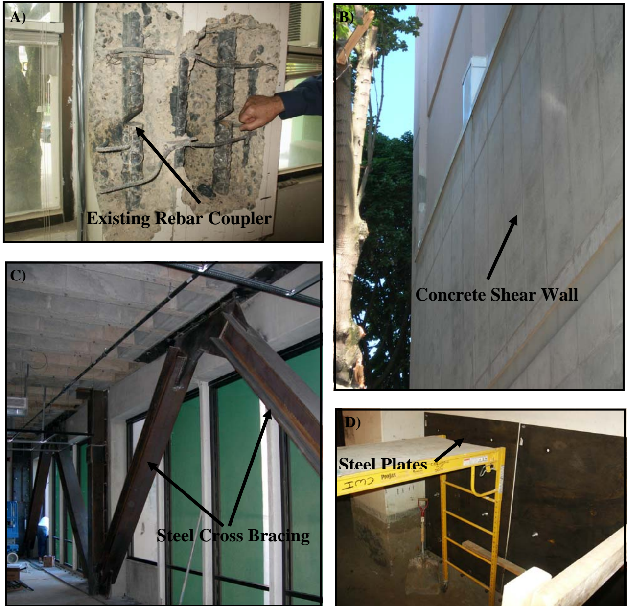
Figure 2. Seismic rehabilitation solutions (A) identifying rebar coupler location in existing concrete columns (B) exterior shear wall addition (C) interior steel cross-bracing, and (4) interior steel plates.
