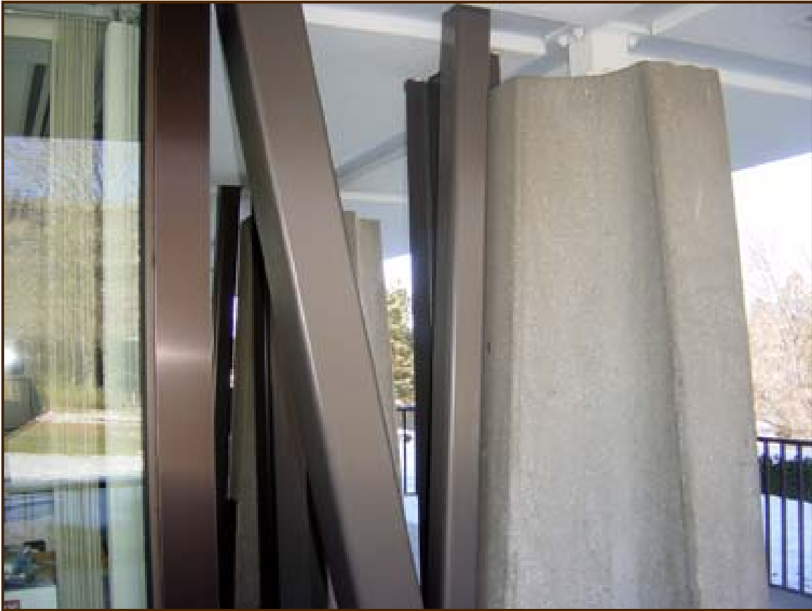
Figure 3. New steel tube bracing to the existing structure on the ground floor to strengthen the building's short direction.
