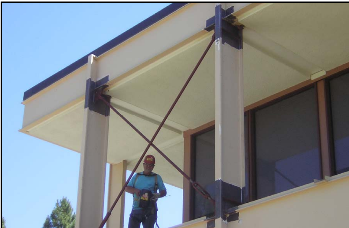
Figure 4. New steel rod diagonal bracing on the 2 nd story to help in the building's long direction
