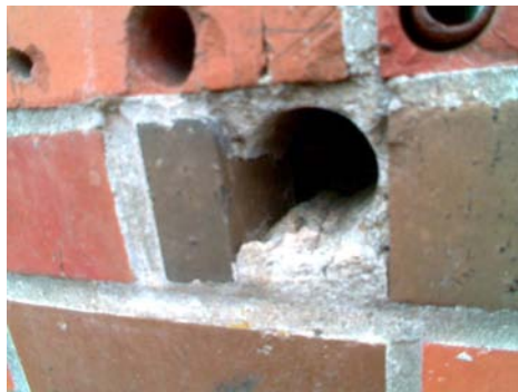
N Primary Structural Type Possible cavity wall, behind first layer of brick some concrete can be seen inside the hole
