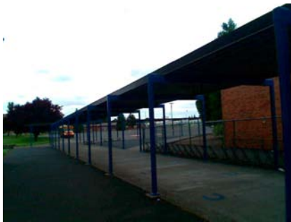
S Falling Hazard
