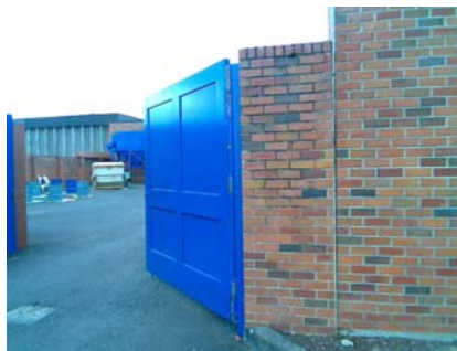
N Falling Hazard Wall disconnected at gap.
