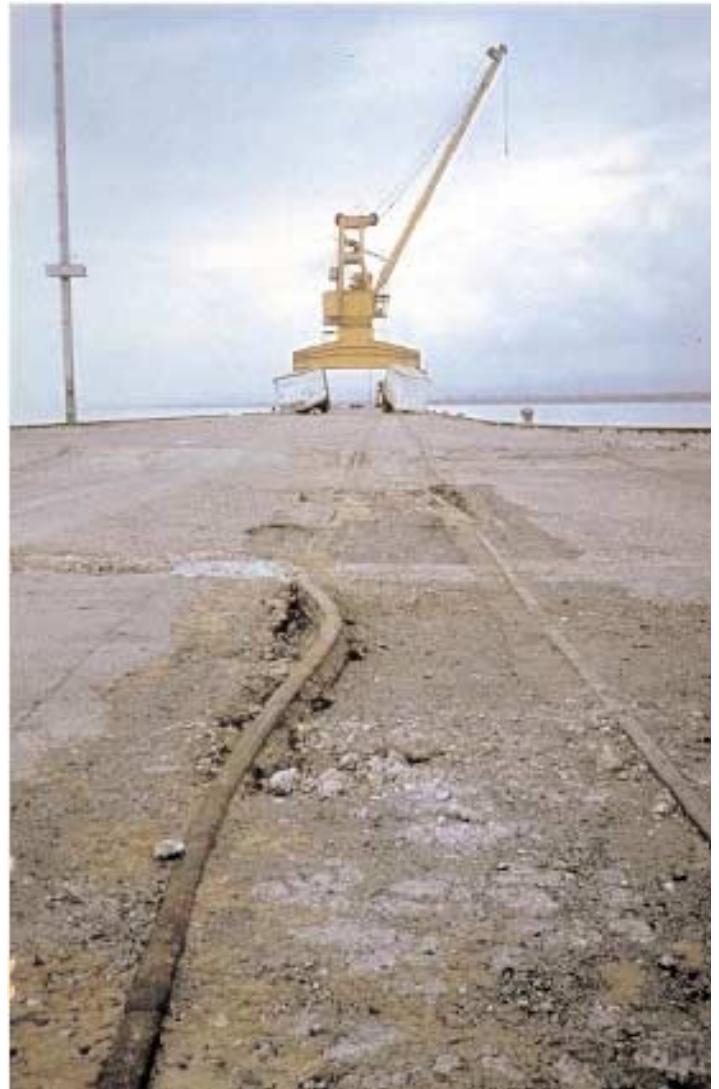
A 1991 earthquake in Costa Rica (M 7.5) damaged rail lines and containers but left the pier and crane undamaged. (Photo from Earthquake Engineering Research Institute)
