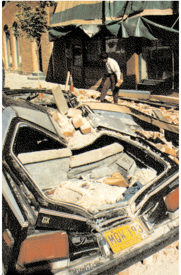
The 1993 earthquakes in Klamath Falls (the strongest were magnitudes 5.9 and 6.0) caused this damage, when falling bricks from an unbraced parapet crushed this automobile parked in front of Swan's Bakery. Photo by Lou Sennick. © Klamath Falls Herald and News, reprinted by permission.
