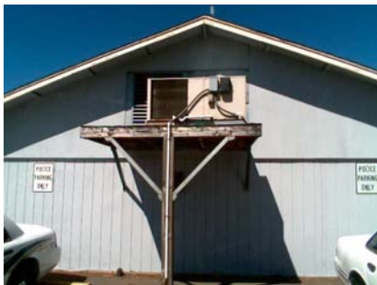
N Falling Hazard
