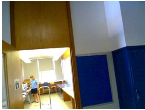
NE Primary Structural Type drywall in the hallway, no shearwalls. Possible Lateral resistant in one direction
